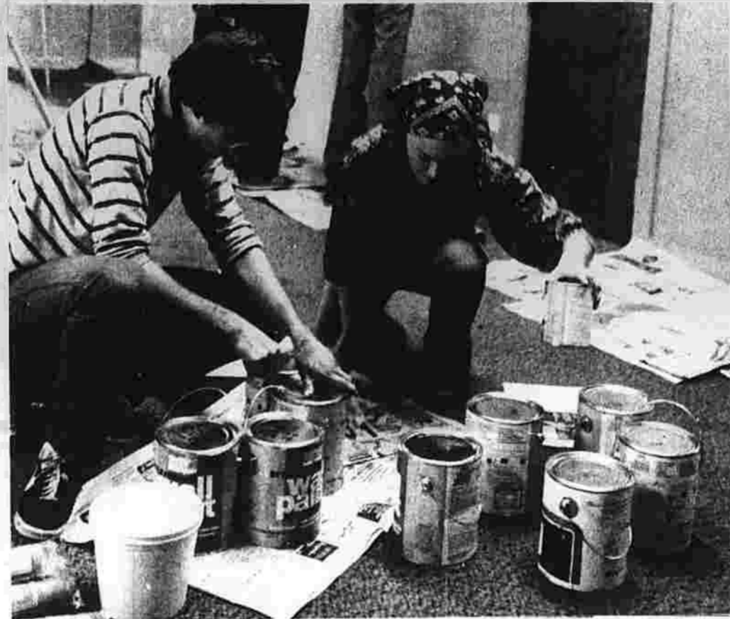
David Tabatsky and Carol Hansen, staff members of Arts Encounter, mix colors for wall paint during a renovation project at their new quarters on Purnell Place. Other staff members are busy painting one of the partitions. (Herald photo by Pinto)
